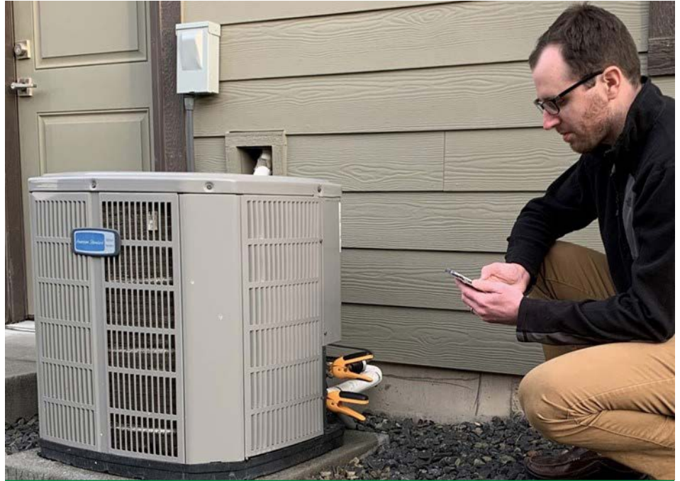
An example of HVAC Smart Diagnostic Tools.
